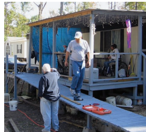
Bob Fousch (left) and Laren Tushim of Alex Semel Council 12989 in Lacombe, La., supervise the construction of a wheelchair ramp while Joseph McDermott (right, background) looks on. McDermott is a veteran of the Vietnam War who was wounded in combat and uses a wheelchair. When McDermott received a new scooter to aid his mobility, Knights built a wheelchair ramp at his home to help him get from the front door to the driveway.
