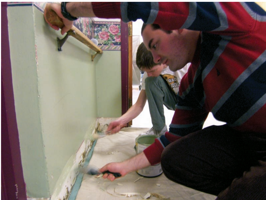
Juan Carmona (right) and Alan O'Connor of John Paul II Council 14188 at Harvard University in Cambridge, Mass., scrape old paint from the baseboards at the Vernon Hall Nursing Home. Knights gathered there each week to paint the facility's laundry room, staff offices and hallways.
