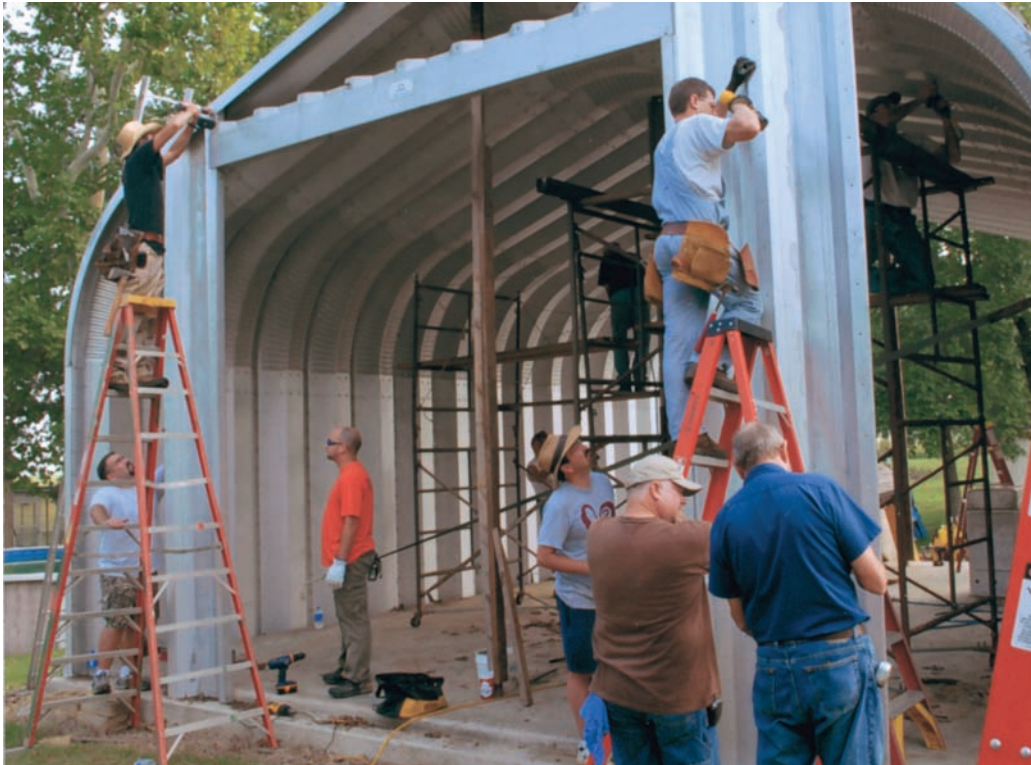
Members of Charleston (Ark.) Council 12875 work to construct a workshop at the home of Brian King, a council member currently serving with the U.S. Armed Forces in Iraq. King began work on the building before his deployment and hoped to finish it upon his return. Aware of the unfinished structure, council members completed the workshop before King arrived home.
