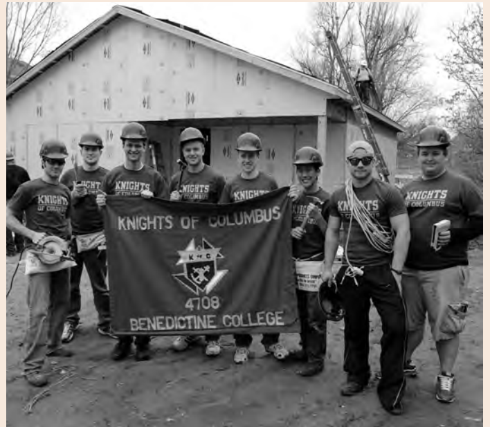
Ten members of St. Benedict's College Council 4708 in Atchison, Kan., joined other volunteers for a Habitat for Humanity project in St. Joseph, Mo. The Knights helped shingle the roof and put up exterior plywood walls.
